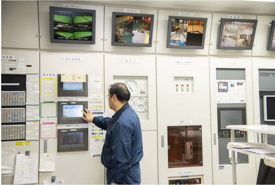
Professional staff members work in the Control Room around the clock.
