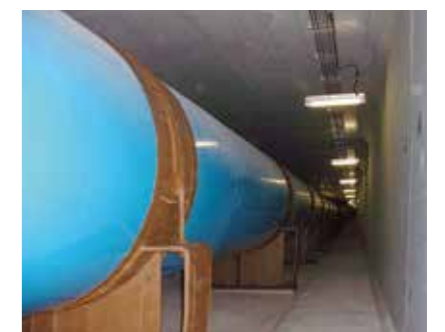
1,350 mm-diameter water pipe
