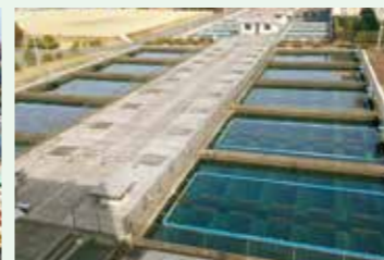
Rapid Sand Filtration Basin
